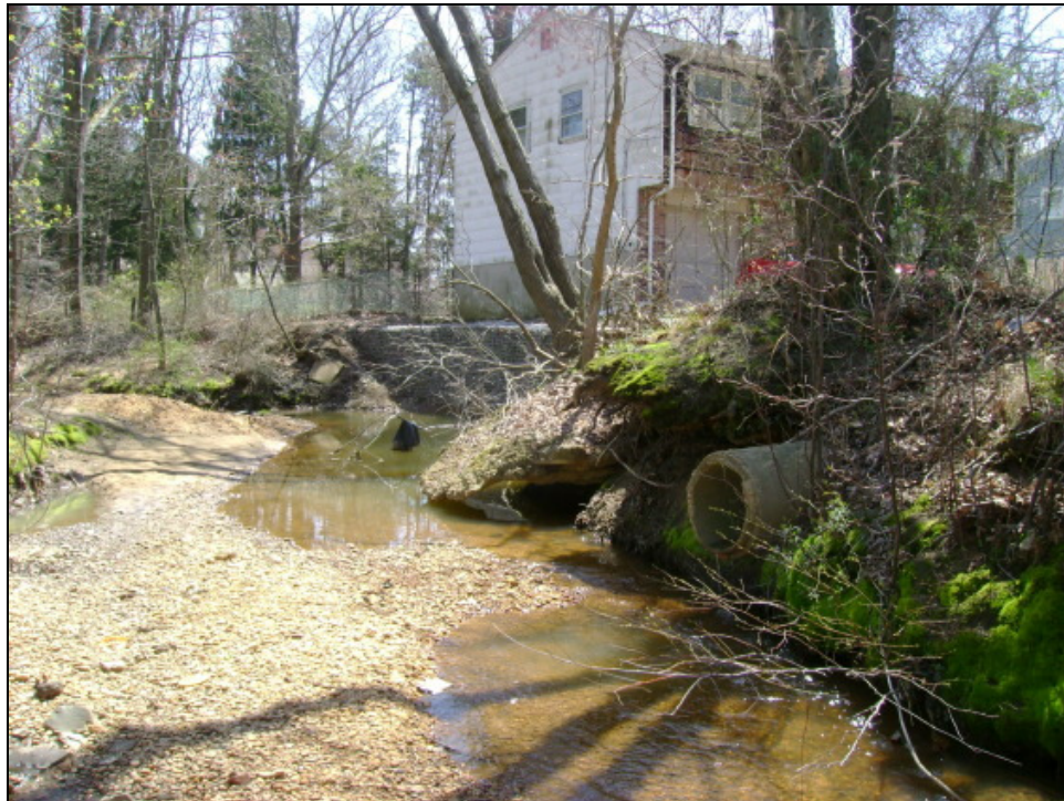
Figure 29. Station #32 looking upstream at street outfall and gabion wall.
