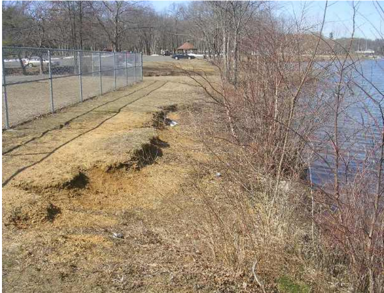
Figure 53. Project section along southern Manalapan Lake shoreline, photo taken facing west, photo taken in January 2010.
