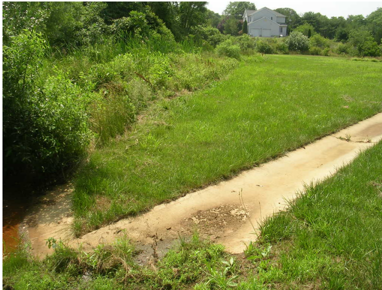
Figure 57. Dry detention basin at station #80, showing turf grass vegetation and concrete low-flow channels, photo taken in summer 2009.
