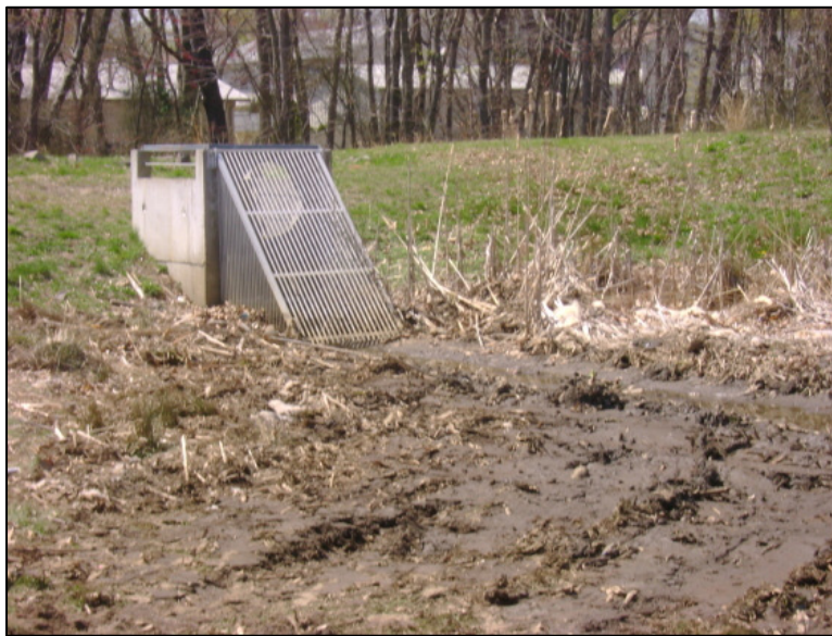
Figure 54. Detention basin at station #32 showing outlet control structure and concrete low flow channel, photo taken in summer 2008.
