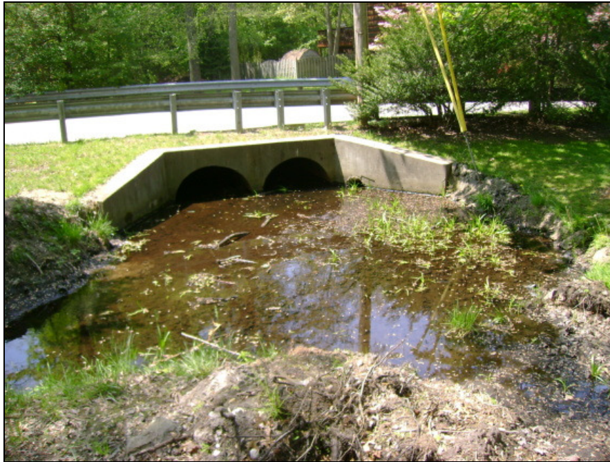
Figure 33. Sediment-clogged culverts at station #3.
