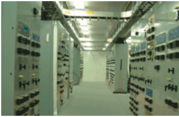
Figure D-4 Substation Control Room
