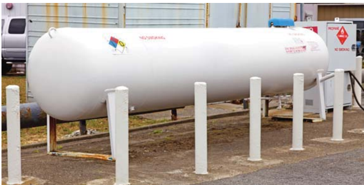
Figures D-4, a-e Various propane facilities
