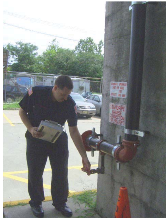
Figure B-3: Local Fire Prevention Bureaus can request assistance from the Division of Fire Safety Bureau of Code Enforcement.
