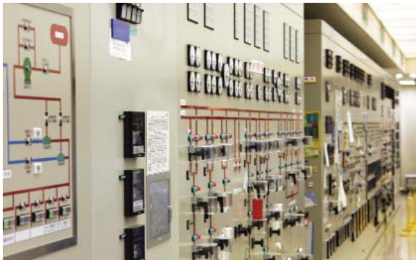
Figure D-5 Substation Control Room
