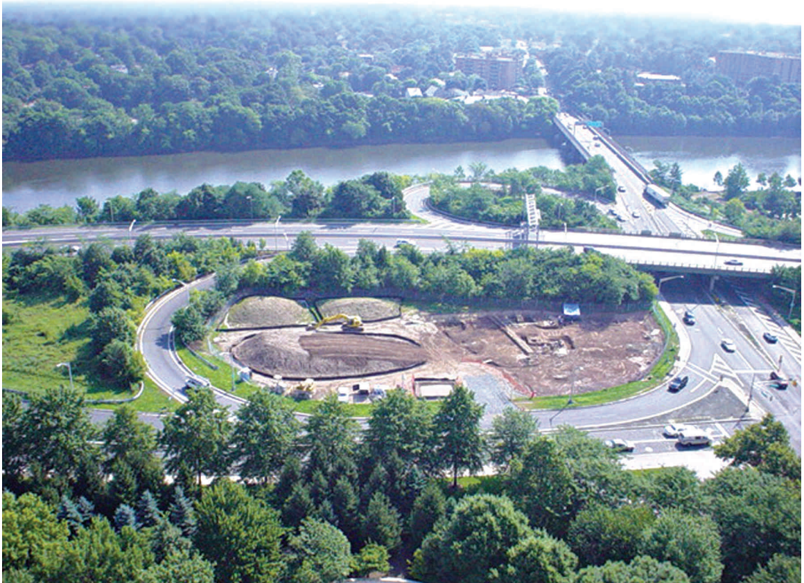
Plate 1. Overhead photograph of Route 18/27 Interchange site from the roof of Johnson and Johnson International Headquarters. Photo by Shane Whilden, 2003.
